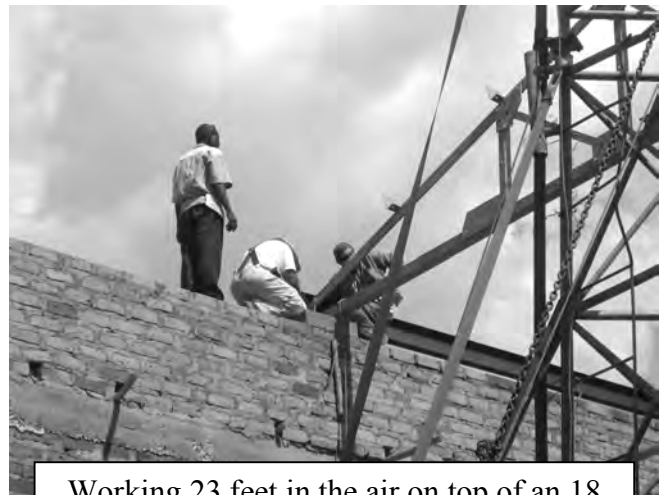
Working 23 feet in the air on top of an 18 inch wide wall.
