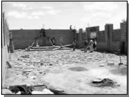
The walls are going up on the new church building in Gungu, Tanzania.
